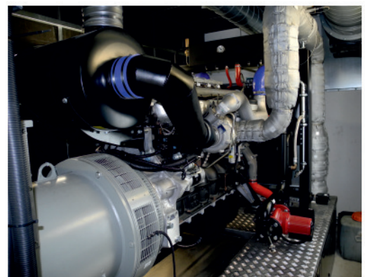
IMES diesel power cogeneration plant
