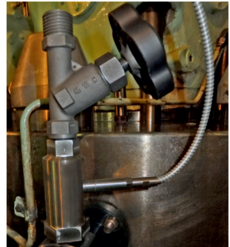
TCS-01CA sensor installed on a MAN&BW two-stroke engine
